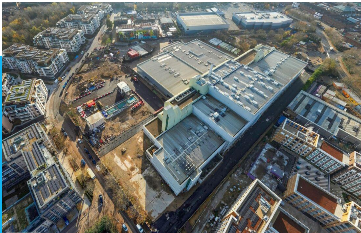
New Haul Road (Printworks Street), Enabling works for Printworks Street and the Printworks building,(November 2023)
