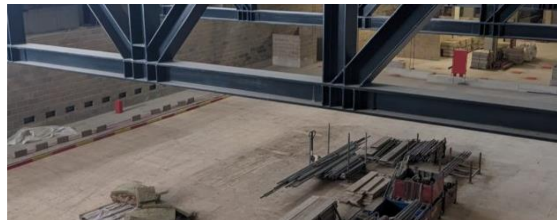
Construction of the new leisure centre and pool for Southwark Council (bottom) and what it will look like (top), June 2023
