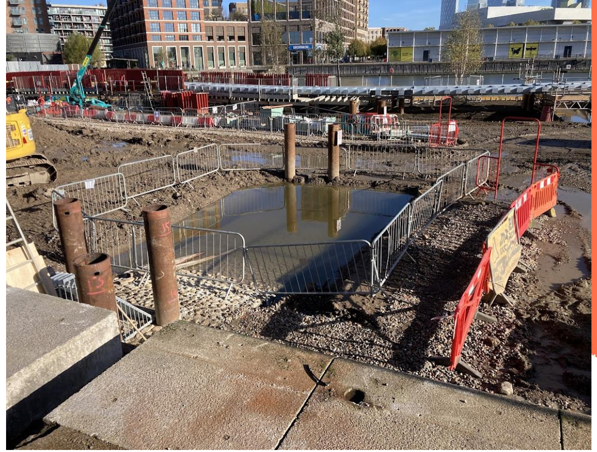
View from Deal Porters Way - SUDs outfall into Canada Dock, January 2024
