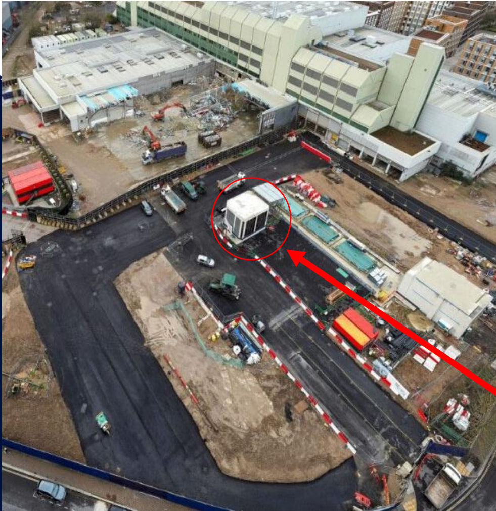
Aerial view of the below ground substation from Quebec Way (December 2023)
